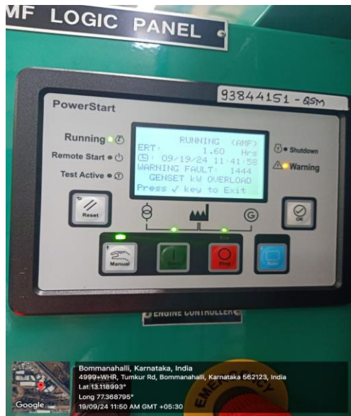
D.G. Control Panel
