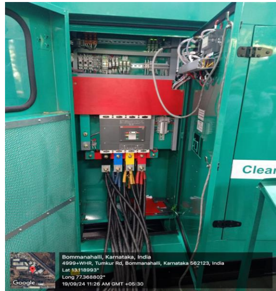
Circuit Breaker - Electrical Output
