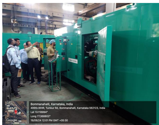
Diesel Generator Inspection and Load Test Images
